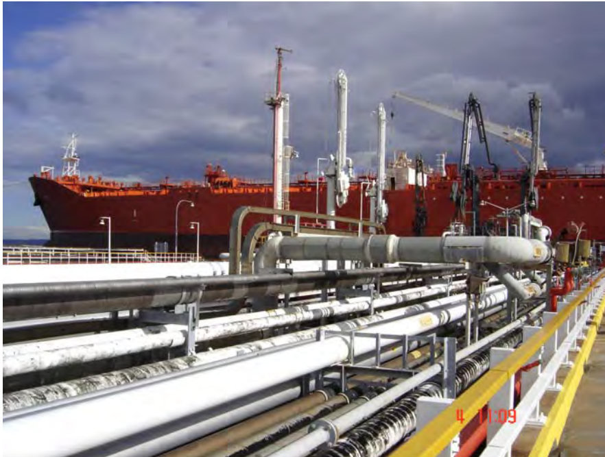
Figure 1-1 View of equipment infrastructure at BLB1
