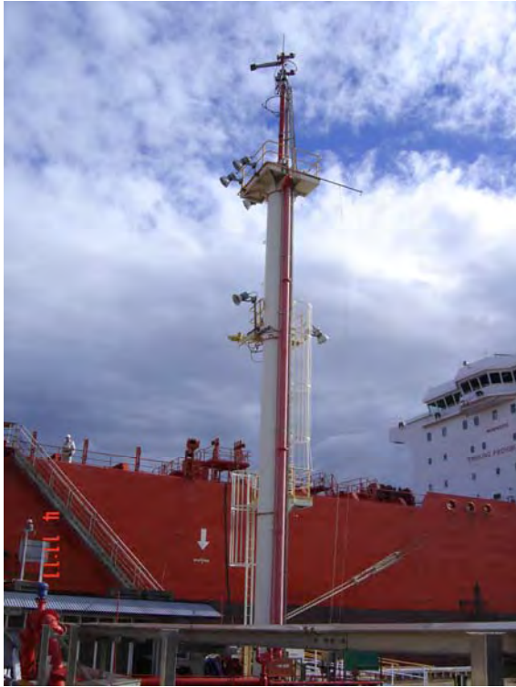
■ Figure 4-6 Existing Fire Monitor at BLB1
