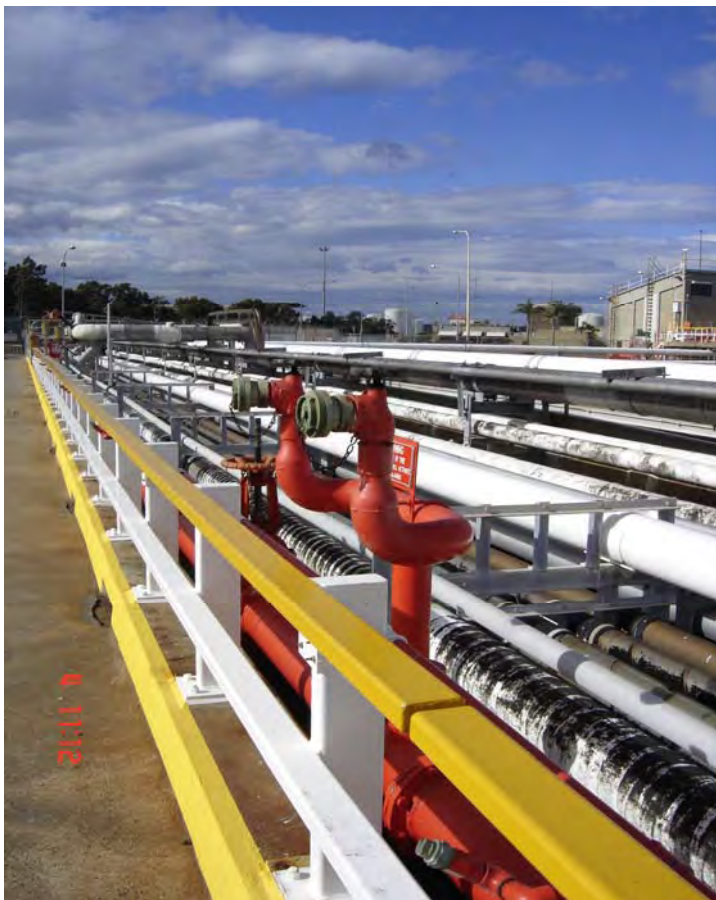
■ Figure 4-7 Existing Pipelines at BLB1
