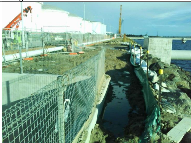
Photo 3 Sediment controls in place adjacent to revetment wall – gap in fence in foreground.
