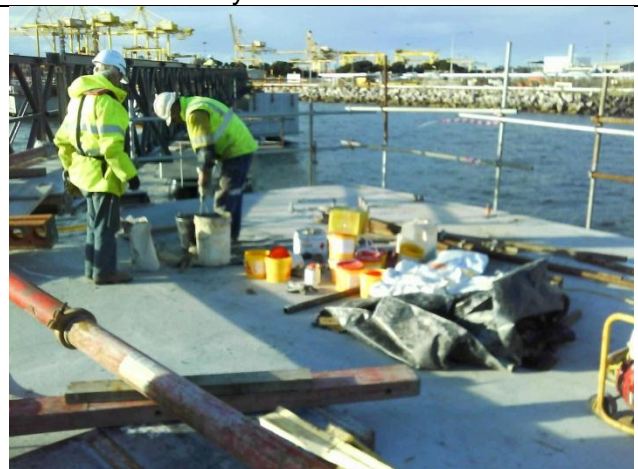
Photo 23 Hazardous substances on working area. There was no secondary containment and no spill kits in the near vicinity
