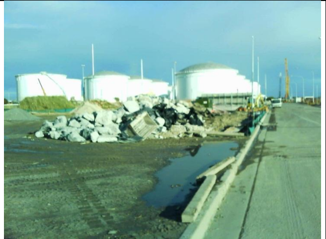
Photo 12 – exit from stockpile area. Tracking of sediment evident.
