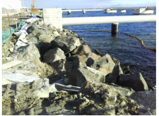
Photo 8 Showing silt curtain around work area and silt fence in need of maintenance
