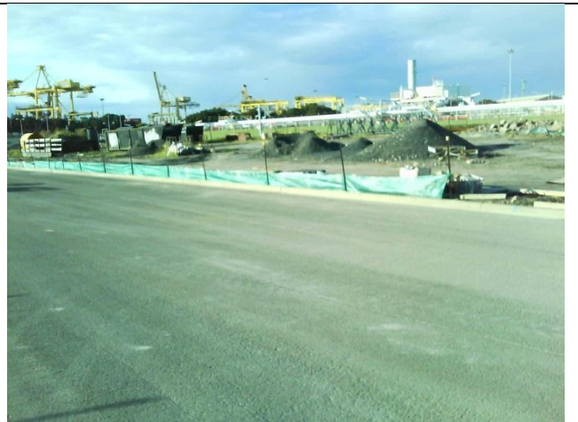
Photo 10 Sediment controls downstream from stockpile area (protection provided for small stockpiles of road base material) in good condition and well maintained
