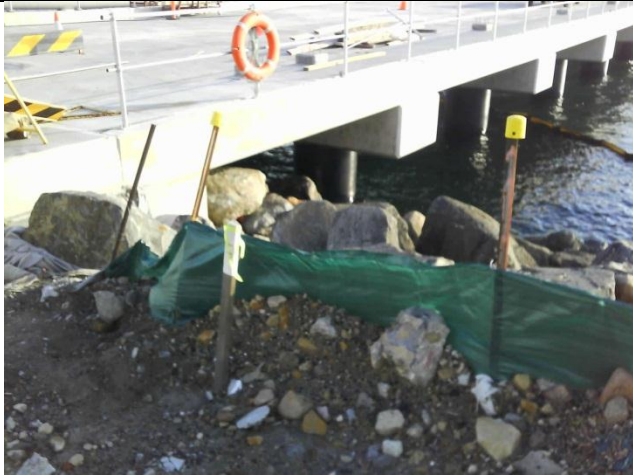
Photo 5 Sediment fence – protection is not continuous
