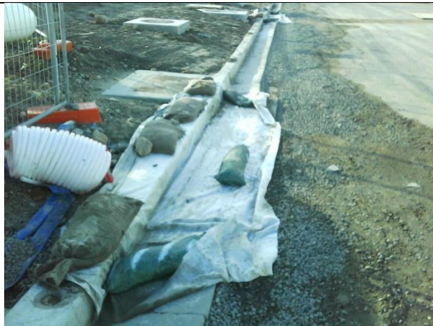
Photo 1 Example of good drain protection measures (however, additional sandbags should be used to hold geofabric down)
