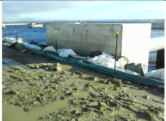
Photo 6 Sediment fence in place – requires maintenance
