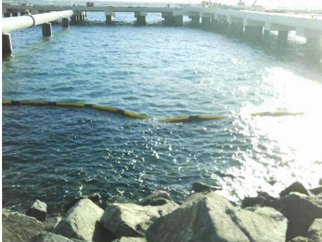
Photo 7 Gap in silt curtain at high tide
