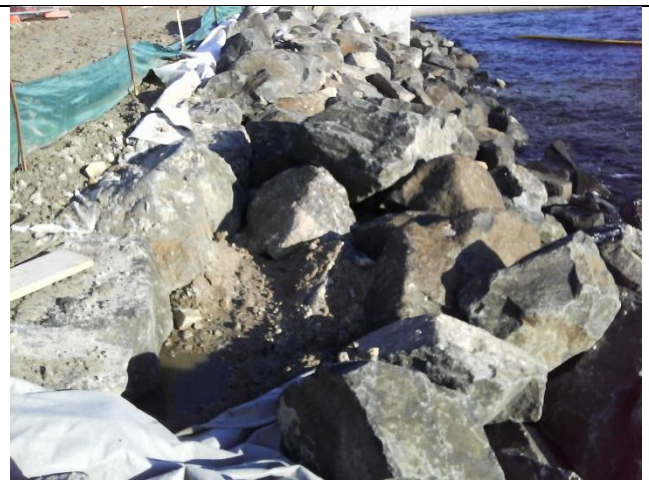
Photo 4 Sediment deposited in revetment wall – appears to be result of washout from sediment fence
