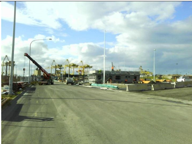
Photo 9 – Sediment controls in place below carpark area – in good condition and well maintained
