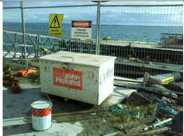
Photo 19 Showing proximity of this area to Botany Bay. There were no barriers / bunding secondary containment between the drums and the water.
