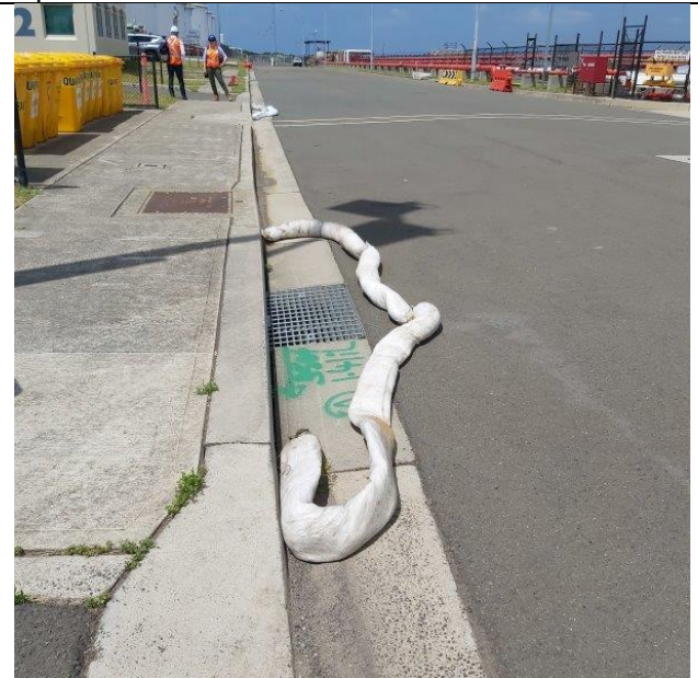
Drains protected by portable oil bunds (identified as vulnerability at previous audit)
