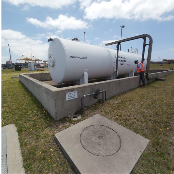
Berth spill containment tank (empty) – fully bunded. Would be used in case of spill at the berth and on site (never used to date)
