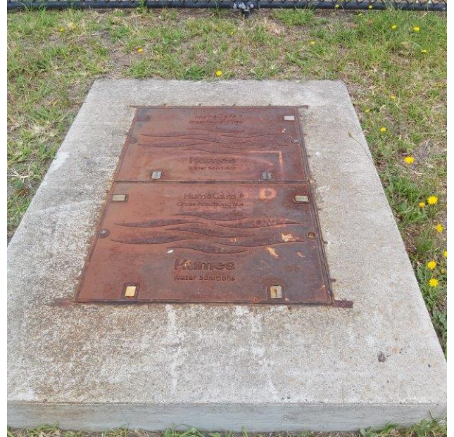
Gross pollutant trap / separator (underground)
