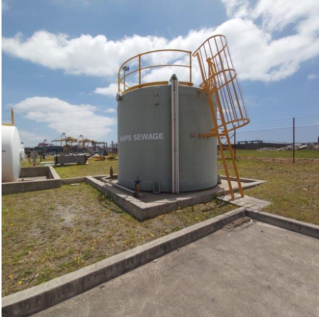
Sewage tank installed to accept ships sewage. The tank has not been used to date and remains empty
