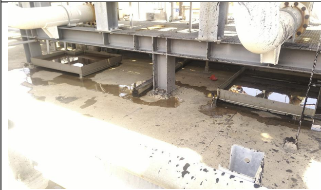
Spill trays full of water – being drained from the tap / valve (potential breeding ground for mosquitos)
