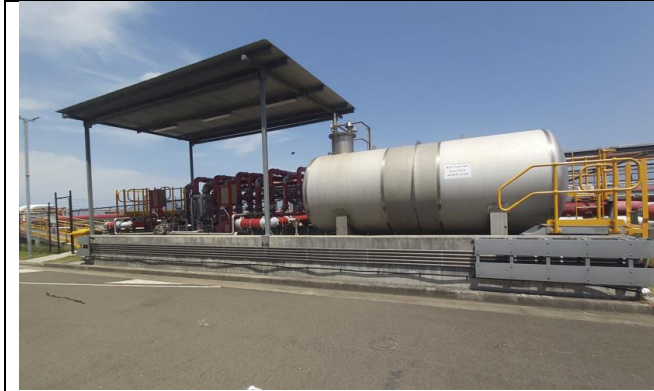
Fire fighting foam tank for BLB2
