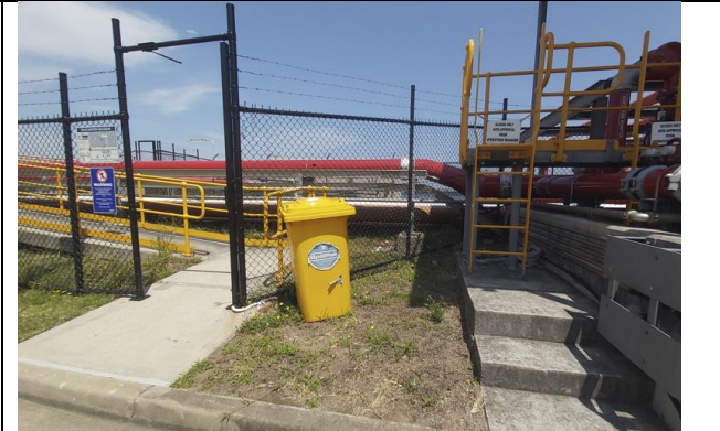
Spill kit stationed near the fire tank and apparatus.
